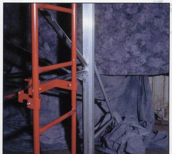
STANDARD SCAFFOLD LADDER FOR SAFE ACCESS TO DECK
